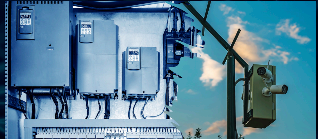
GROUND CONTROL UNIT
